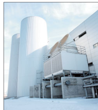
Promoting energy conservation through high-efficiency operation using predictive controls in heat accumulator-type air conditioning
